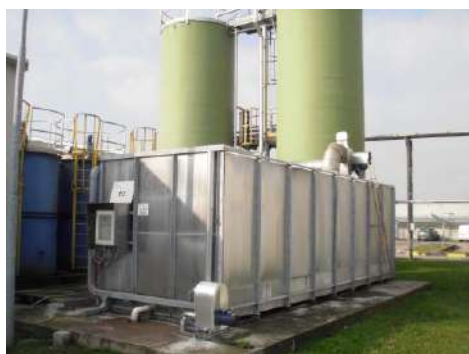
Figura 15: Biofiltro Air Clean, E2
