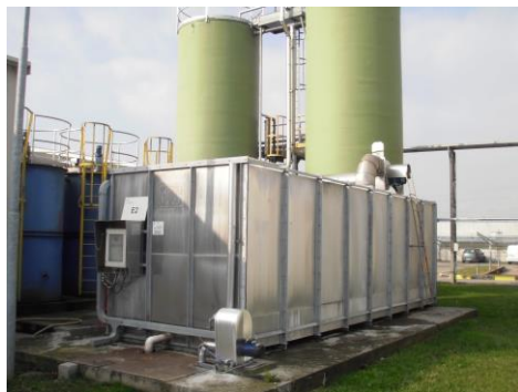
Figura 17: Biofiltro Air Clean, E2
