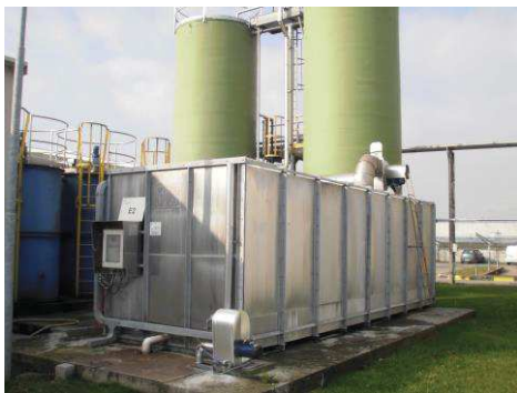
Figura 17: Biofiltro Air Clean, E2
