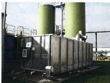
Figura 18: Biofiltro Air Clean, E2
