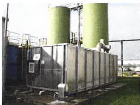
Figura 18: Biofiltro Air Clean, E2
