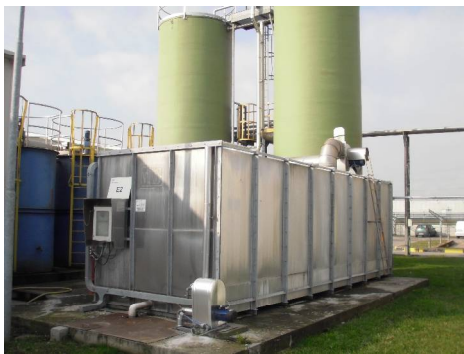
Figura 18: Biofiltro AirClean, E2
