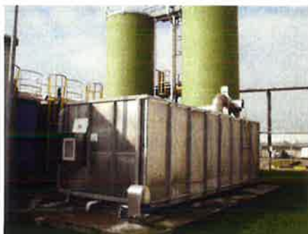
Figura 18: Biofiltro Air Clean, E2
