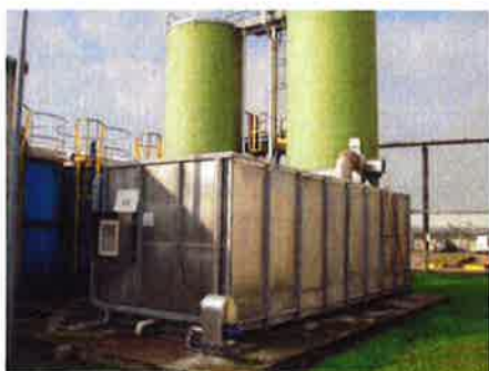
Figura 18: Biofiltro Air Clean, E2
