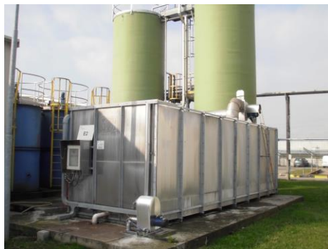
Figura 18: Biofiltro Air Clean, E2
